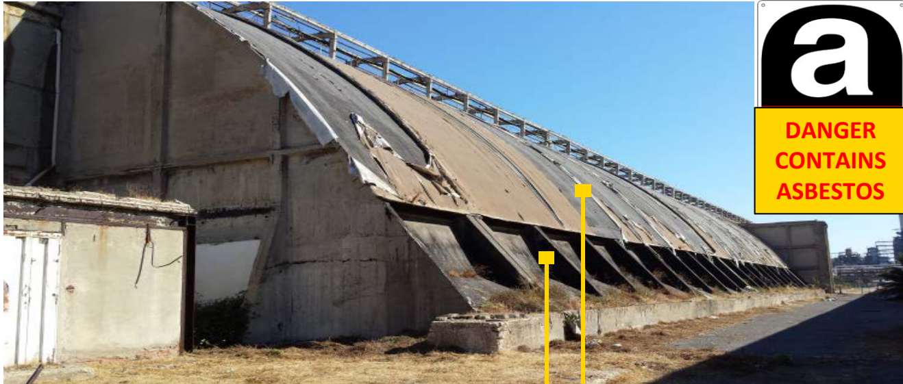
Friable asbestos in waterproofing layer covering the roof and the buttresses
