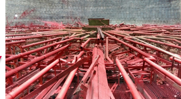
ACM pipes at the bottom of the tower, up to 6 m from ground
