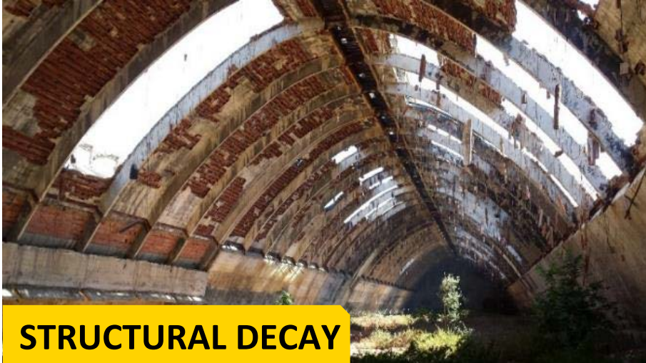
STRUCTURAL DECAY Brick cover partially collapsed
