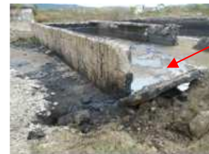
Coal tar spillage
